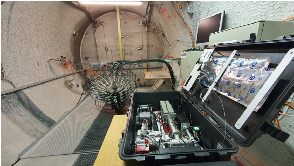
Fig. 3-5: On 13 January 2022, the miniRUEDI acquired by Entracers GmbH was installed at the GTS close to the GAST plug
